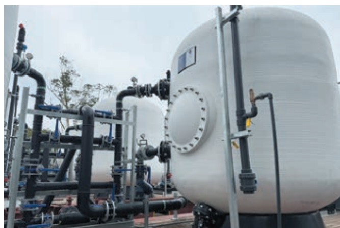
Figure 4: Mobile PFAS treatment unit at Cascade Water Filtration Plant
