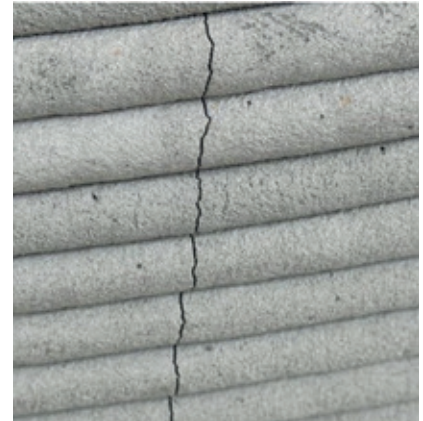
Figure 5: Exterior cracks in 3D printed structure
