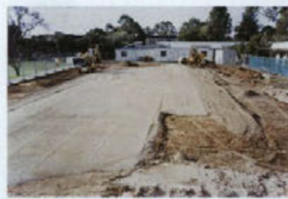
The old Year 5 classrooms were demolished to make way for the new library/resource centre.
