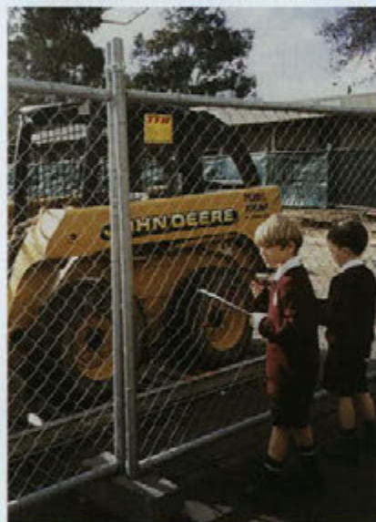
Preparatory School students have enjoyed watching the demolition and building process throughout the year.
